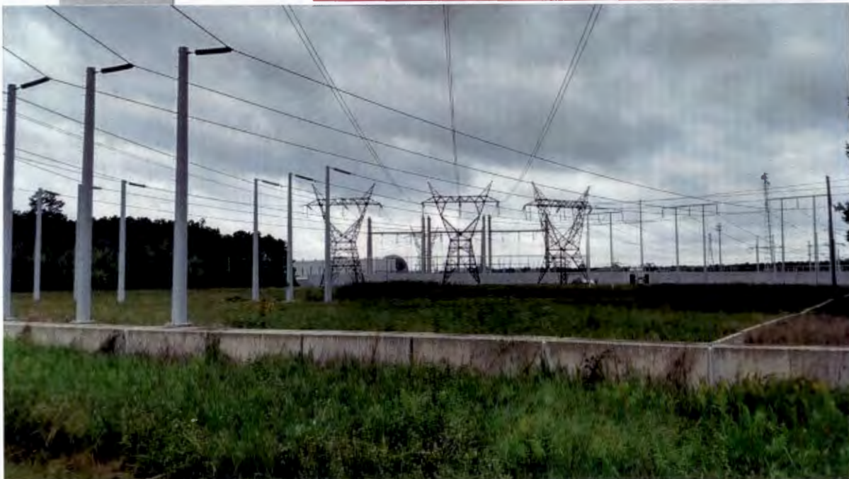
High voltage power lines near Surry Power Station
